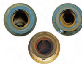
Inlet and outlet of worn pressure regulators.
